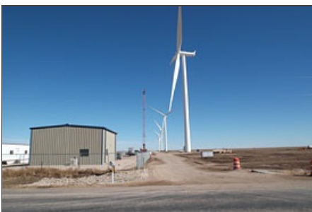
Each of the five new 2.3 megawatt turbines will contribute to the 11.5 MW total generation capacity at the site.
